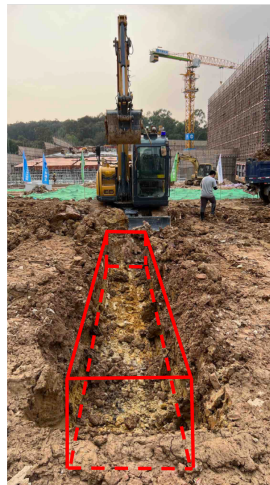
Fig. 6: Autonomous trenching. The goal is to excavate a 1m \times 1m \times 6m area as shown in the red cuboid.
