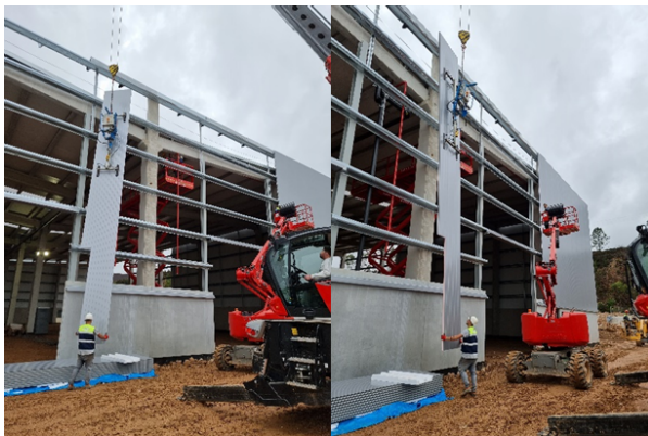
Fig. 3. A high degree of physical interaction is maintained between telehandler and ground worker until the sandwich panel fits in the structure.
